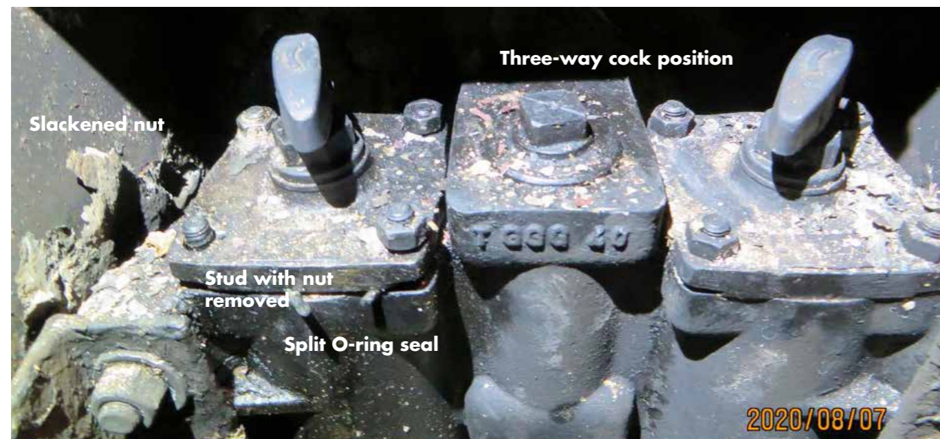
AE1 fuel filters, showing three-way cock position as found post-fire and AE1 left-hand fuel filter cover and split O-ring seal
