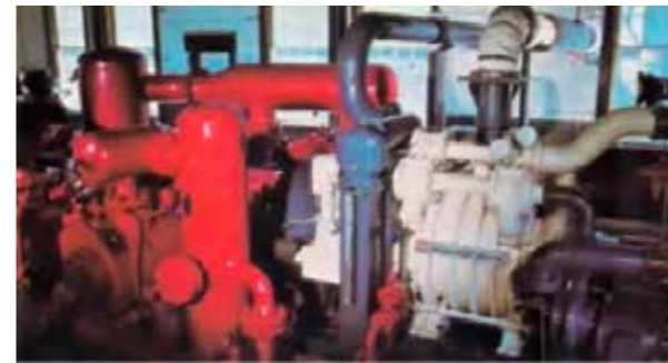
IR5000 engine driving an RDS-2 reciprocating compressor in a Pennsylvania gas boosting installation, c. 1977.
